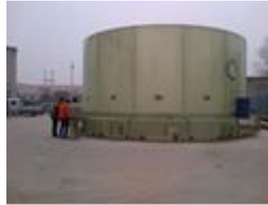
Feedwells & related for WesTech for GE Power Australia
