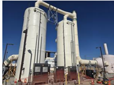
Odor control system for Avondale, Arizona
