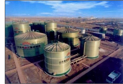
Tank farm of field wound tanks
