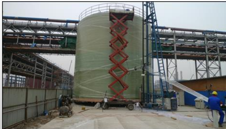
Field wound process water tank Syria
