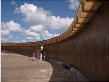
Clarifier liner and internals
