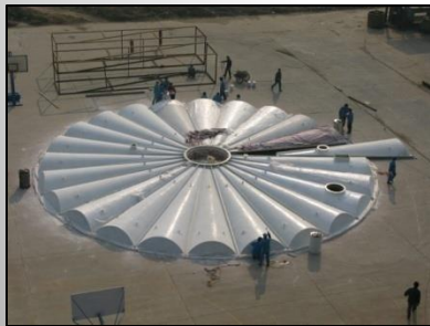
60' dia. clarifier cover
