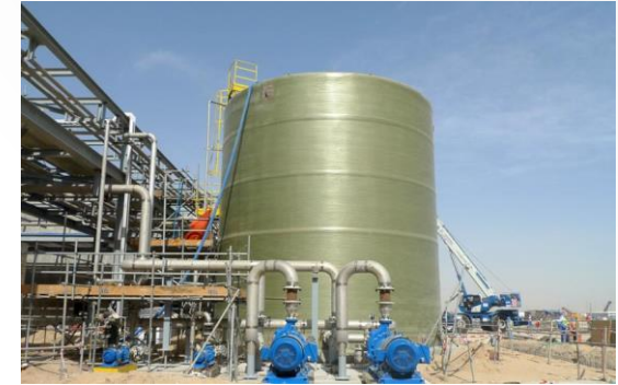
Come into service after hydrostatic test
